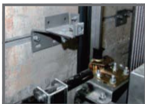
Elevator shaft - guide rail fixings
