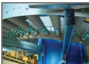
Conveyor system fixings
