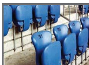
Stadium seat fixings
